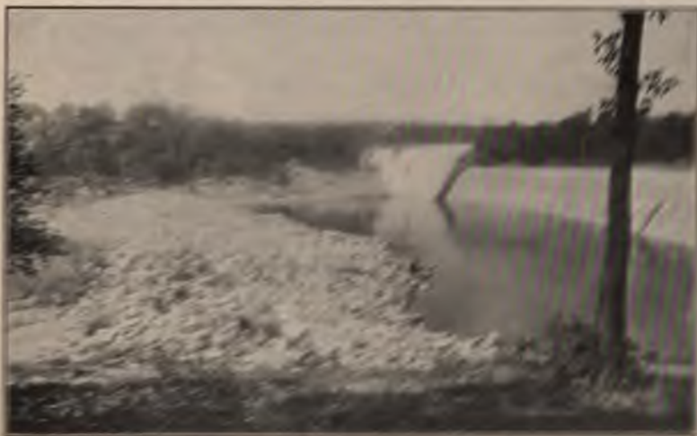
FIG. 25.—Rock erosion below Scioto River storage dam.
